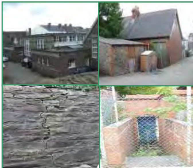
Above: Maintenance Issues at Ysgol Gymraeg Brynmawr
