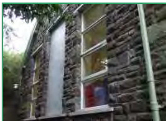
Ysgol Gymraeg Brynmawr ; maintenance Issues
