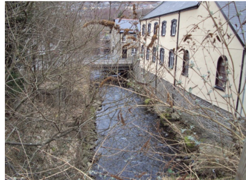
Plate 6: Ebbw Fach River and Chapel Road bridge, looking upstream (north) from headwall of the culvert
