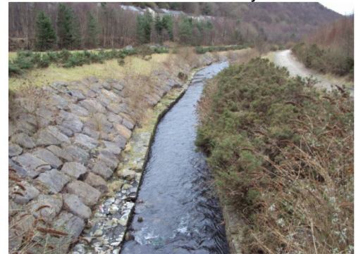
Plate 4: Ebbw Fach River at culvert outlet, to the south of the site, looking downstream (south)
